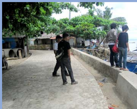
▲ DAVAO : This sea-front embankment built by the SAJUSSA community (106 households) with only a $750 small project loan from ACCA, has helped to stop some serious coastal erosion. The city has taken up the idea and is continuing the embankment along the shoreline.
