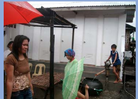
▲ TALISAY : The SALUPA community (150 households) used a $3,300 loan from ACCA and $300 worth of building materials from the local government to build this new communal toilet block with hand pumps, to replace a broken-down municipal toilet nobody could use.
