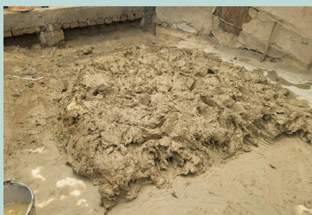
Mud mixed with husk and cow dung was applied to bamboo walls in Jeetpursimara to enhance insulation.
