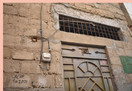
Low-cost improvised solutions to improve air circulation are common in Karachi.
