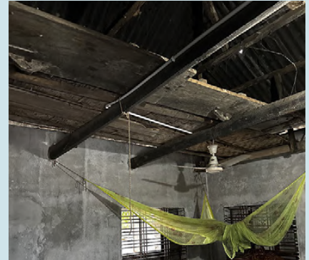
Wooden planks under the roof as a heat barrier.
